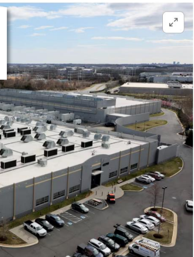
[1/5] A car drives past a building of the Digital Reality Data Center in Ashburn, Virginia, U.S., March 17, 2025.
